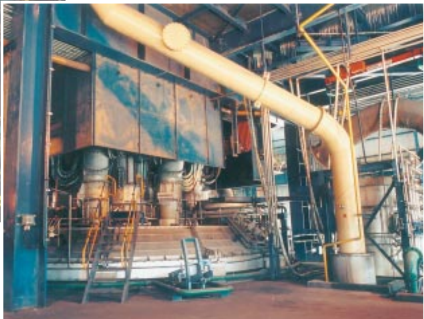
The roof of the furnace with the Bateman Titaco electrode system and the feed chutes.
