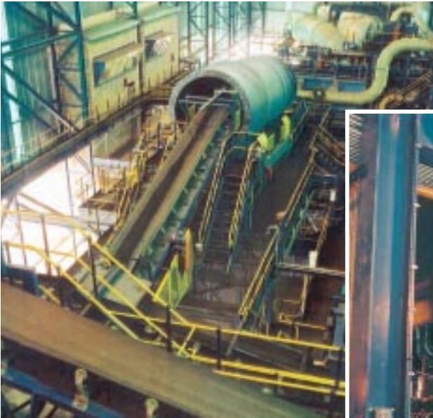
The Assmang sinter plant.
